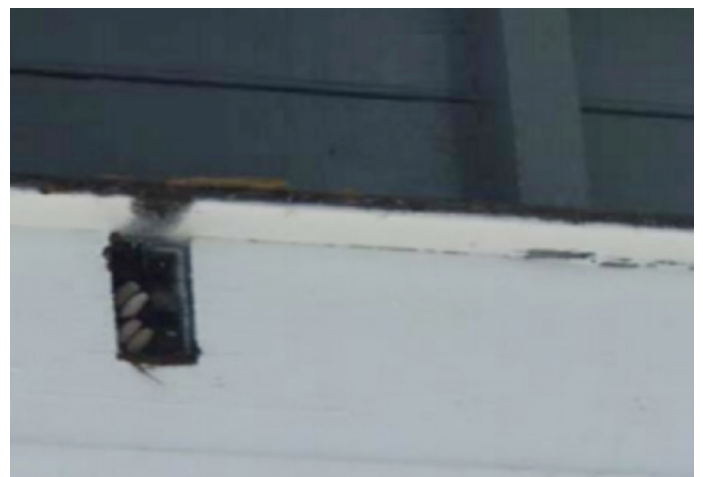
Mud wasp nests in the bearer housing is evidence that a sizeable gap existed where the floor joist cog was not fully engaged into the bearer
