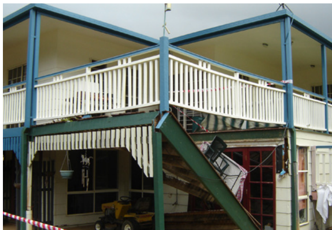
Collapsed corner of the deck is clearly visible in these photographs
