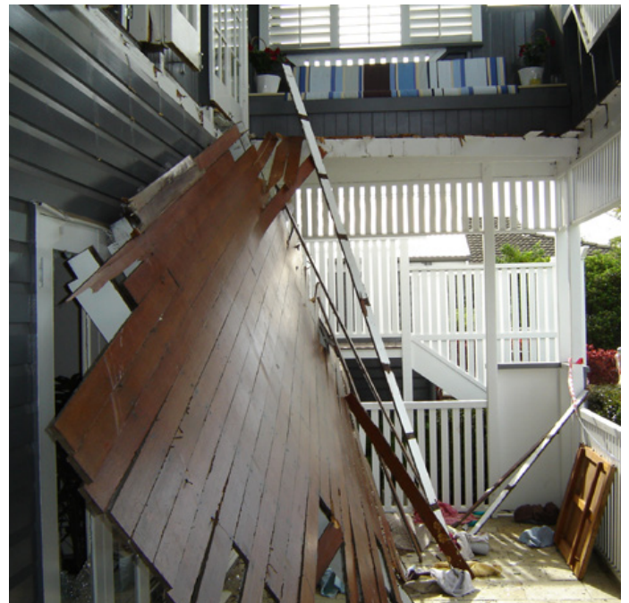
View of collapsed deck
