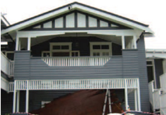
Ascot residence subject to balcony collapse
