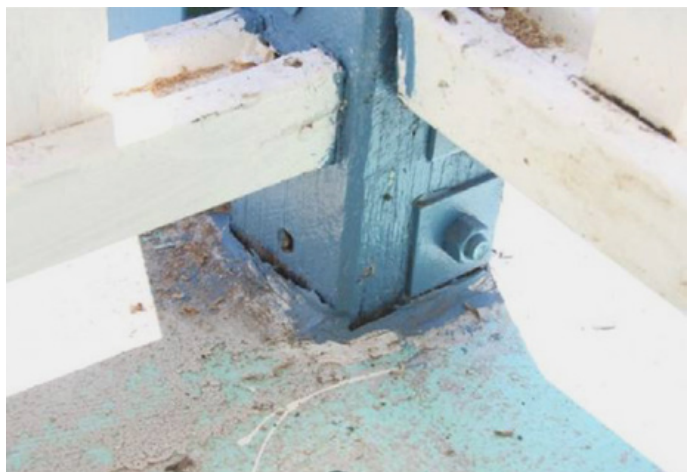
Gaps around base of veranda post allow water ingress into wall cavity
